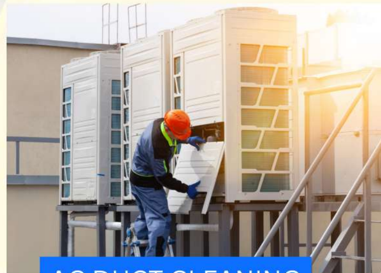
AC DUCT CLEANING
